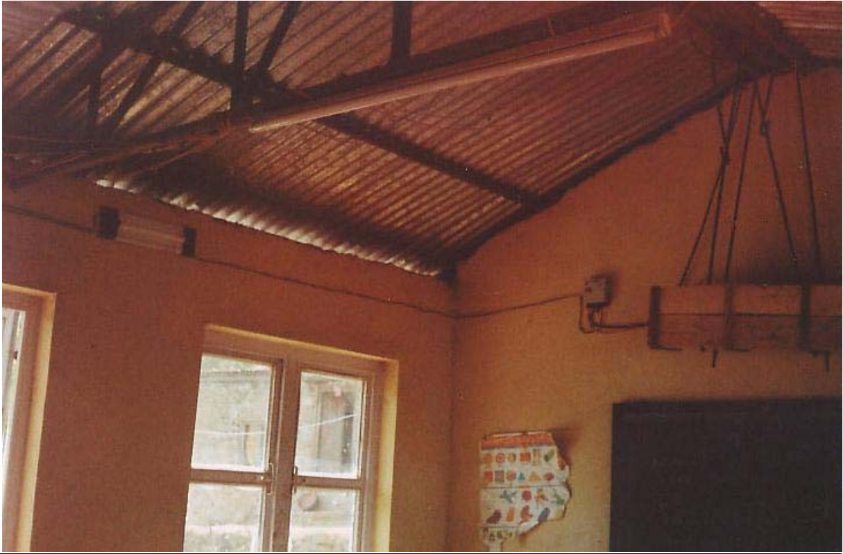
Fig 5: TL Lamp and Charge Controller Connection
