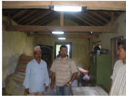
Fig. 5: Lights operating after Successful Completion of Installation
