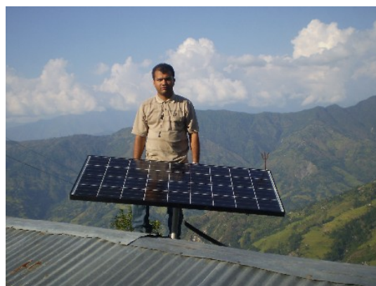
Fig. 3: Panel and lightning Arrester
