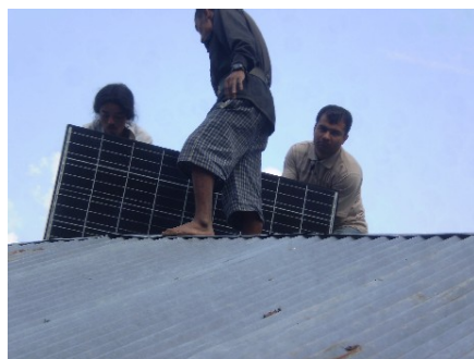
Fig. 2: Lasersun Technician and Umbrella Guys working together for the Installation of Solar Photovoltaic System
